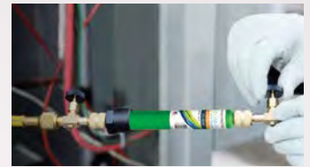
Charge inline with refrigerant
