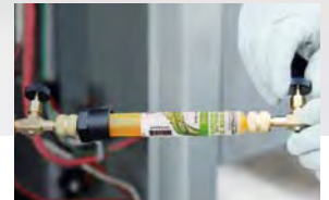
Charge inline with refrigerant
