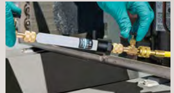
Charge inline with refrigerant
